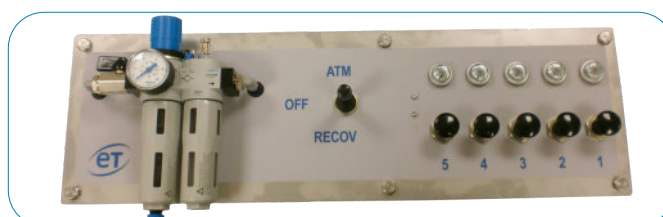
5 Compartments panel with filter-regulator and vapor recovery control
